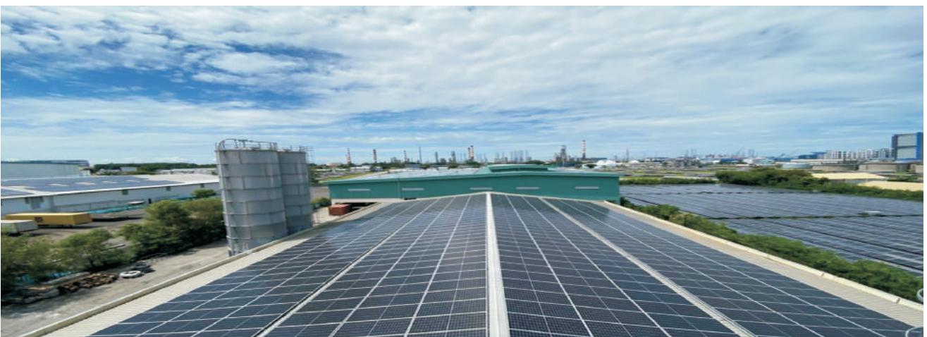
Singapore Roof 870KW
