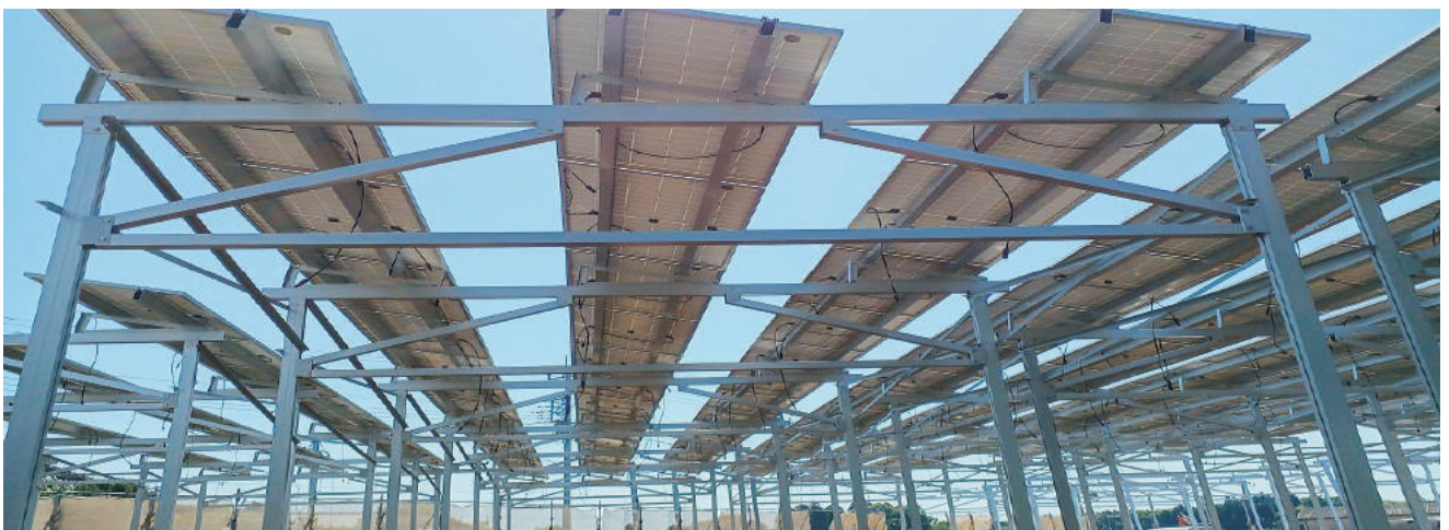
Chiba Prefecture Solar Sharing Mounting System 1.3MW
